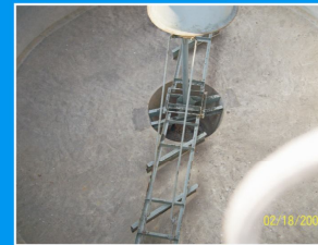
Centrally Driven Clarifier Mechanism
